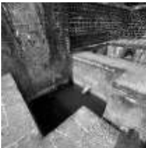
3 Stage Water Tank System at Ranjeshwar Temple, Ranje, Tal. Bhor, Dist. Pune
